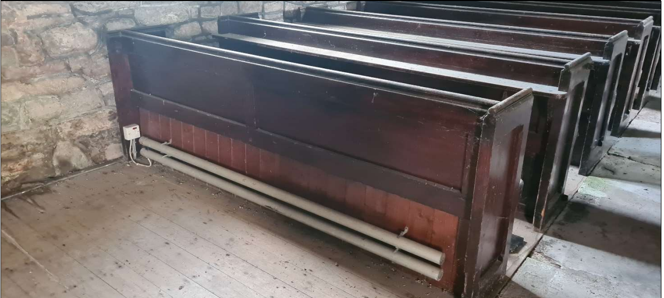
Electric tube heaters fixed to pews.
